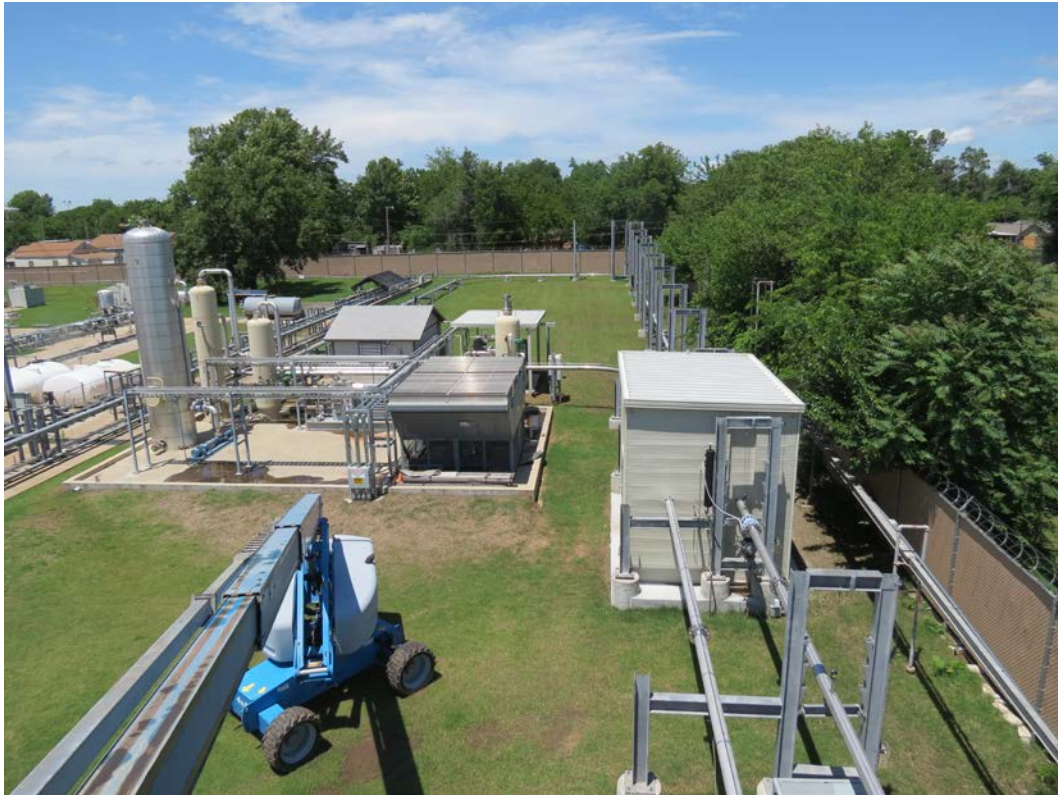
Figure 3. View of 6-in. High Pressure Large-Diameter Pipeline Flow Loop
