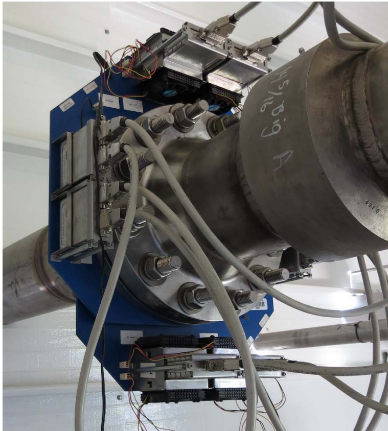
Figure 1. Dual WMS installed at 6-in. High Pressure Large-Diameter Pipeline Flow Loop.
